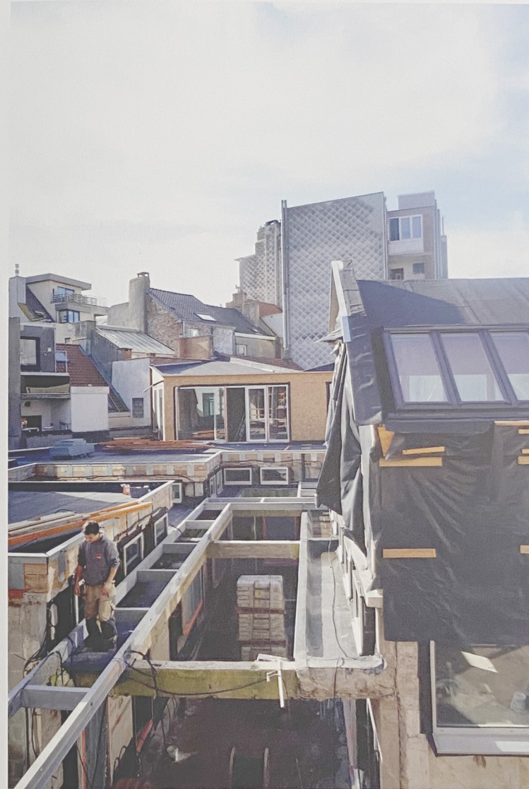
View of the exterior during construction, showing the existing structure and some of the new additions
